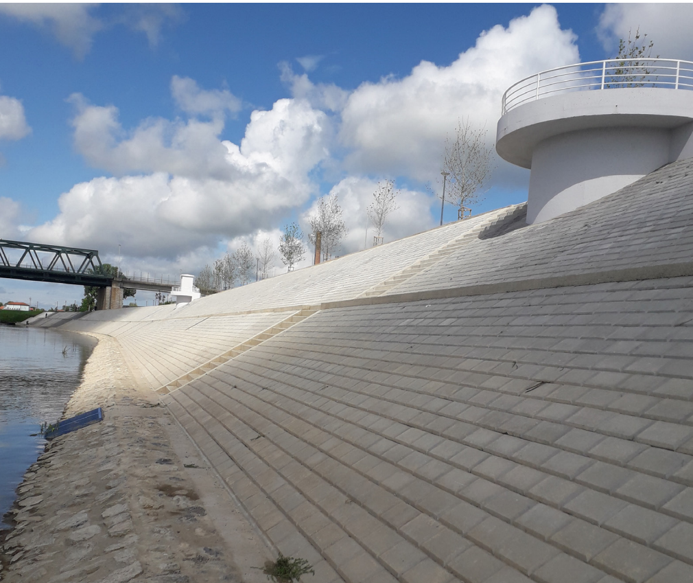
Picture 6. Construction of the riverbank protection on the left bank of the Sava River in Slavonski Brod co-financed by a CEB loan
