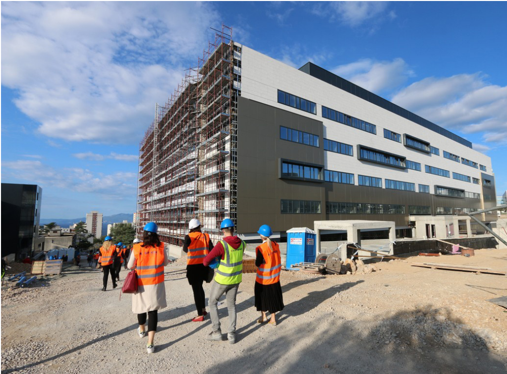
Picture 7: The construction site of the new KBC Rijeka hospital in the Sušak area is co-financed by loans from the CEB (Council of Europe Development Bank).
